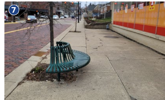
Sidewalks near the Family Dollar store have some cracks in the pavement but are overall in relatively good shape. Streetscaping features such as trees and benches provide amenities for pedestrians.
