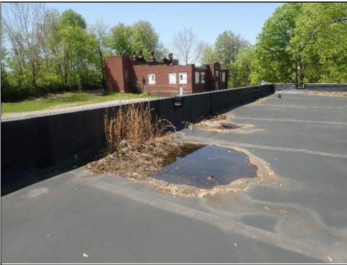
Depressions at structural damage below
