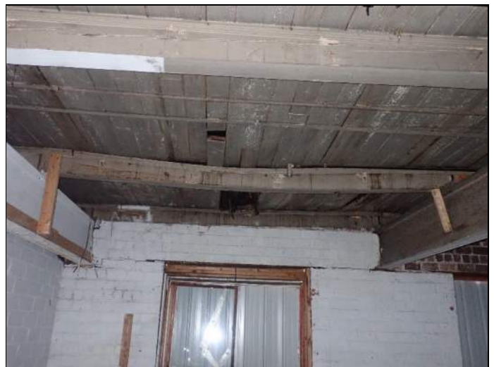
Deflected roof beam
