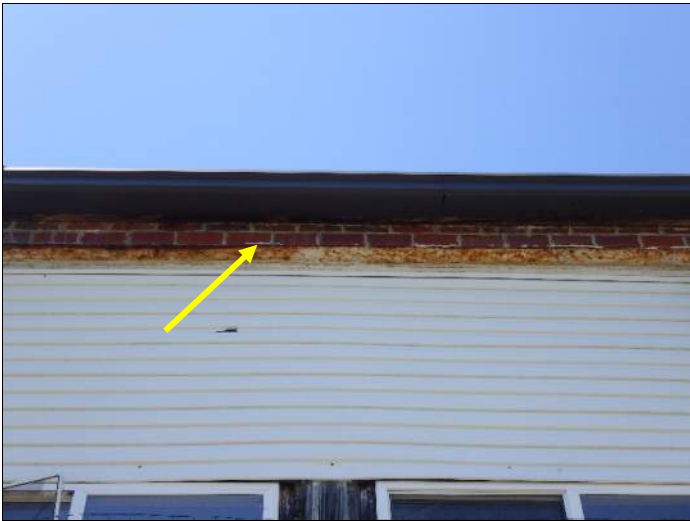
Typical corroded lintel
