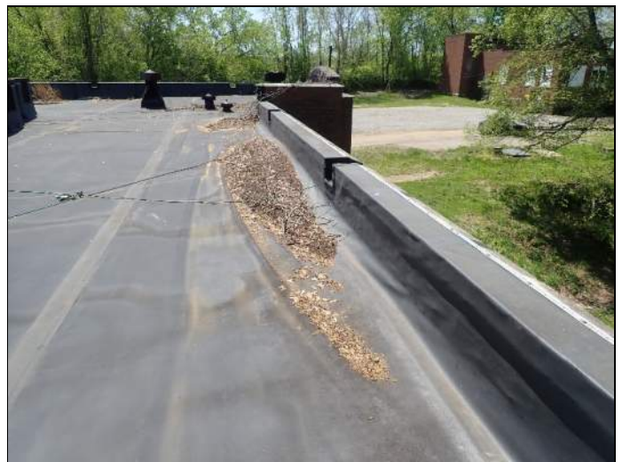
Piles of debris on roof
