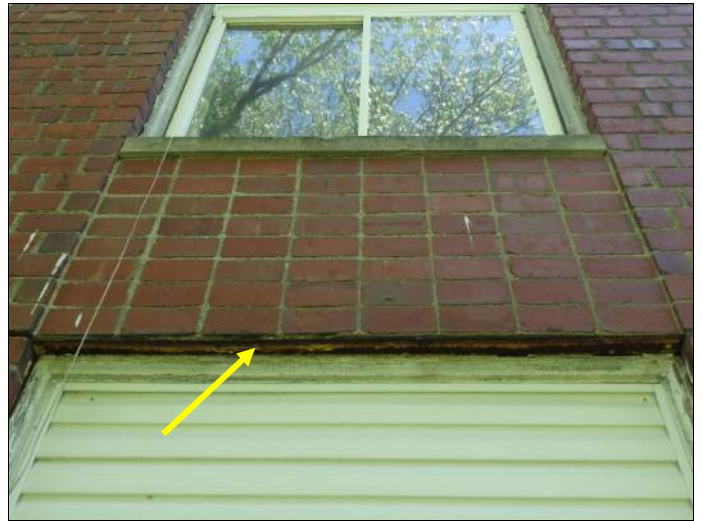
Typical corroded lintel
