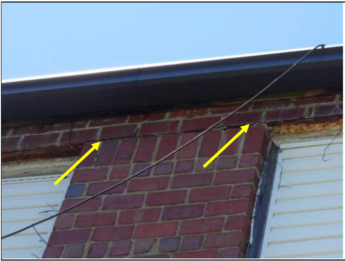
Brick and mortar separation from lintel
