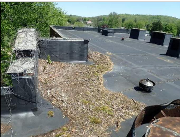
Piles of debris on roof
