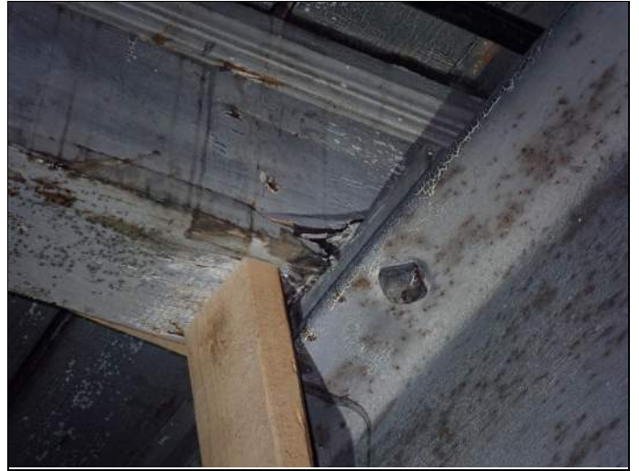
Crushed wood at bearing
