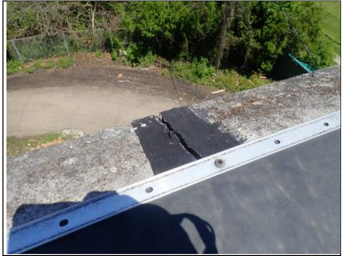
Failed coping joints
