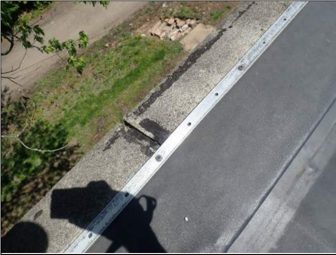
Failed coping joints
