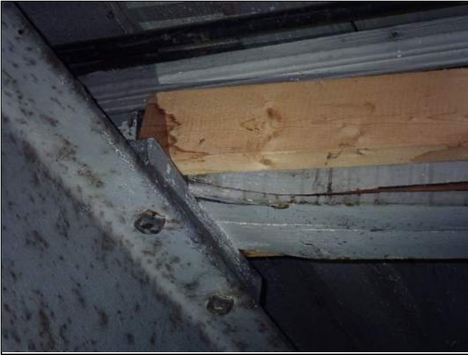
Crushed wood at bearing
