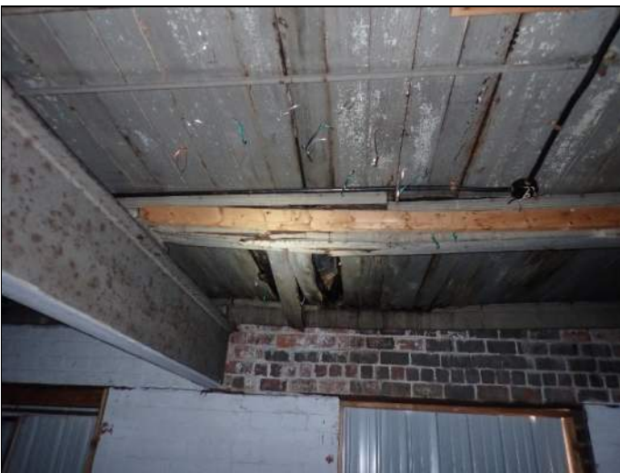
Fractured roof beam and deteriorated roof deck
