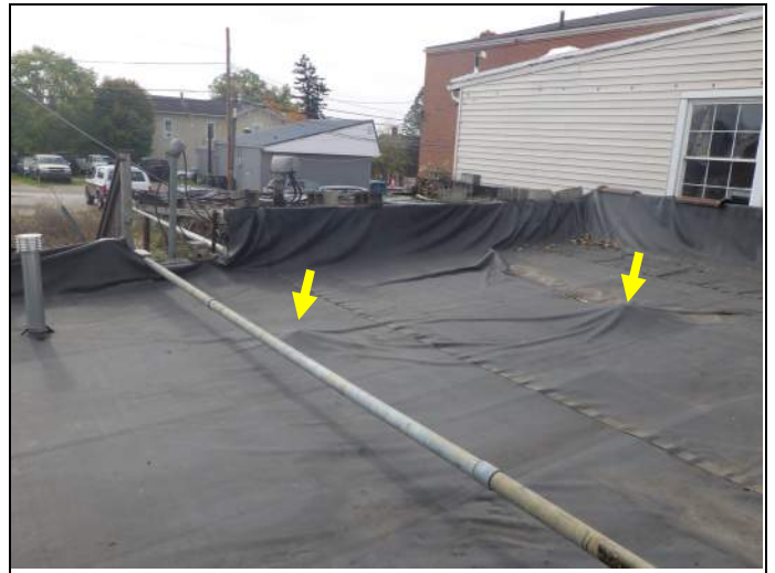
Protruding plumbing below membrane
