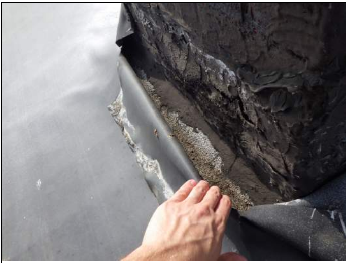
No termination bars or counter flashing at chimney
