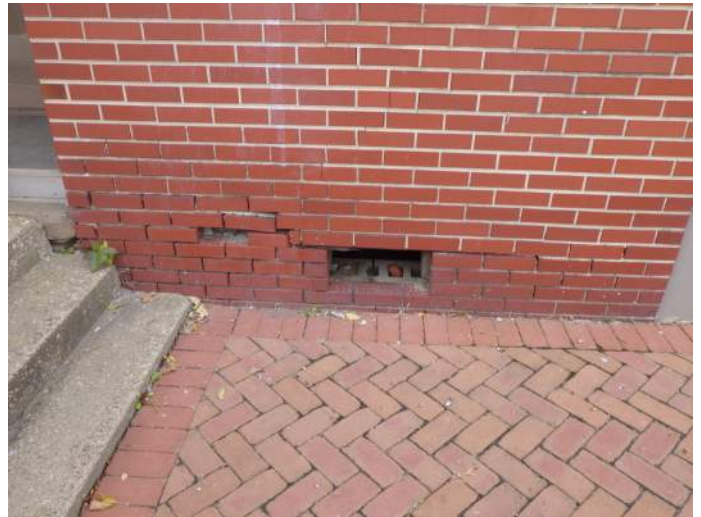
Deteriorated brick veneer and mortar
