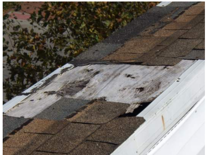
Missing shingles and plywood over parapet
