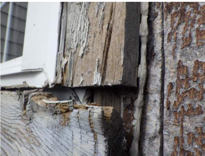
Deteriorated wood trim
