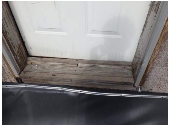
Missing threshold at second-story door
