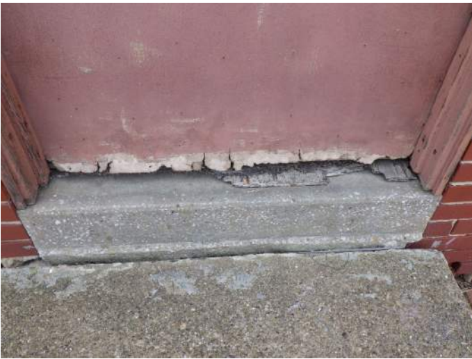
Delaminating wood door
