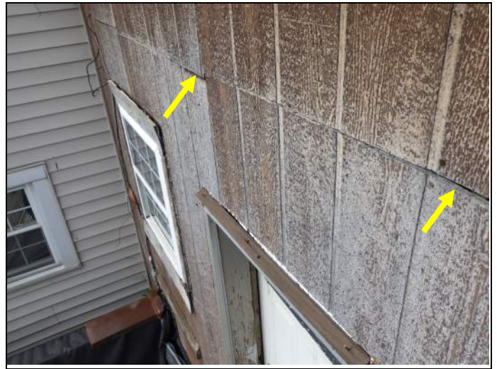
Open joints in T1-11 siding
