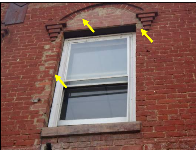
Stair step cracks in brick veneer
