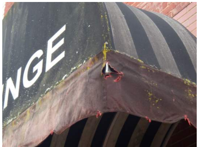
Deteriorated storefront awning
