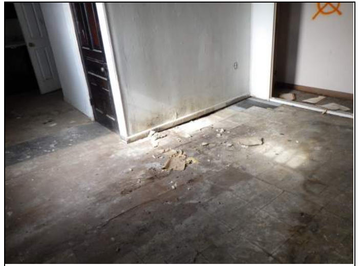
Area below water leak on second story
