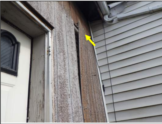
Warped T1-11 siding
