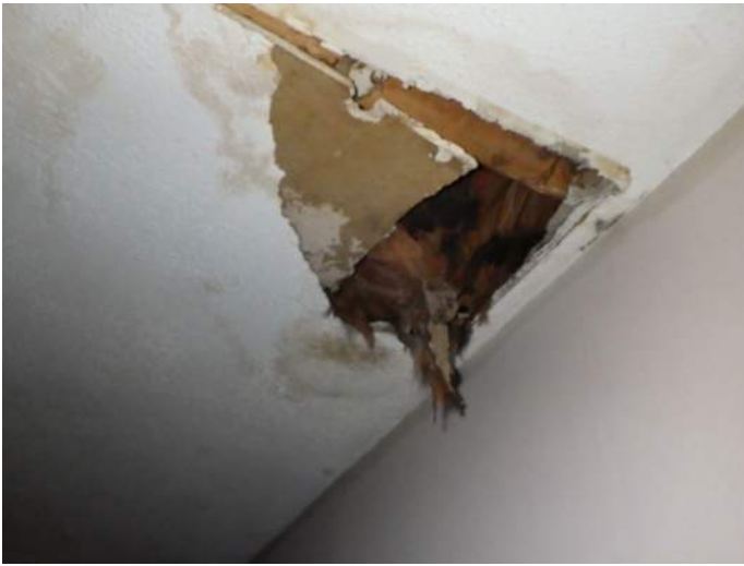
Area of water leak from roof on second story
