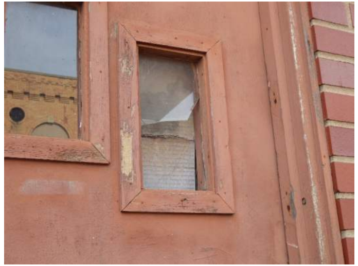
Broken window in wood door
