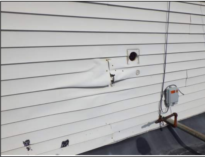
Warped vinyl siding
