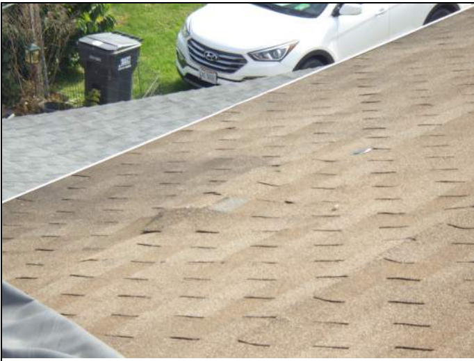
Uneven roof surface
