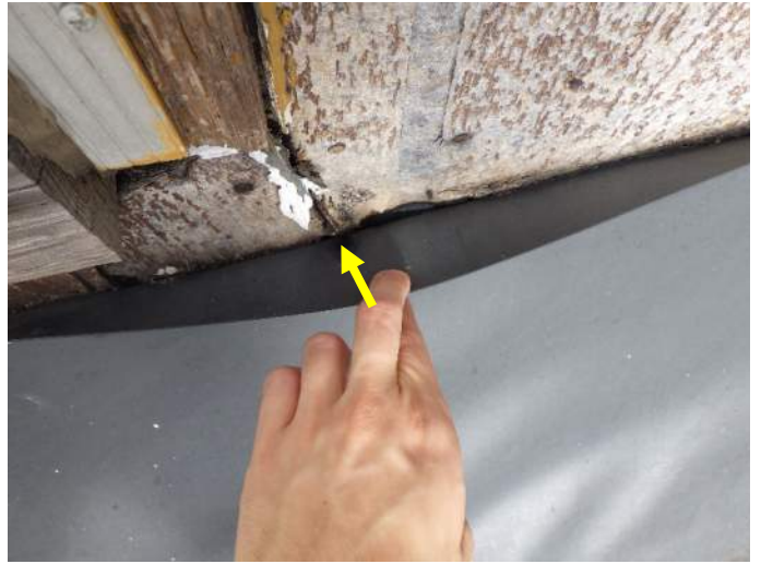
Void at joint in T1-11 siding
