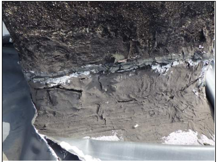
Cracked and deteriorated sealant
