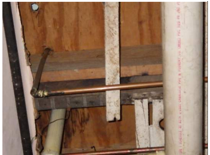
Sistered second story floor joist
