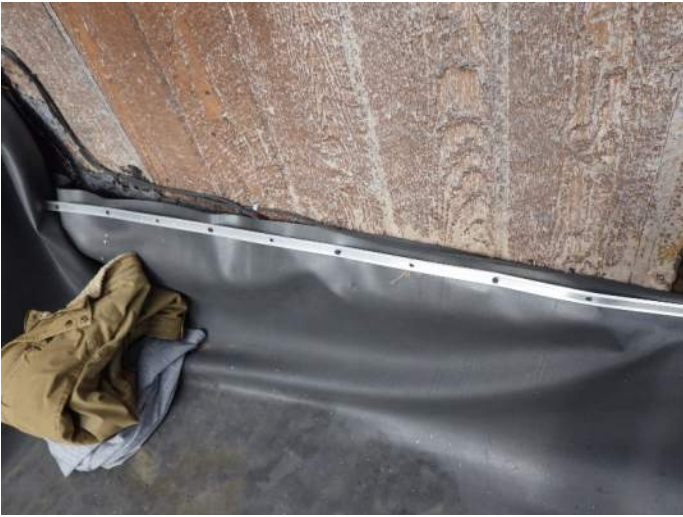
Termination bar along T1-11 siding
