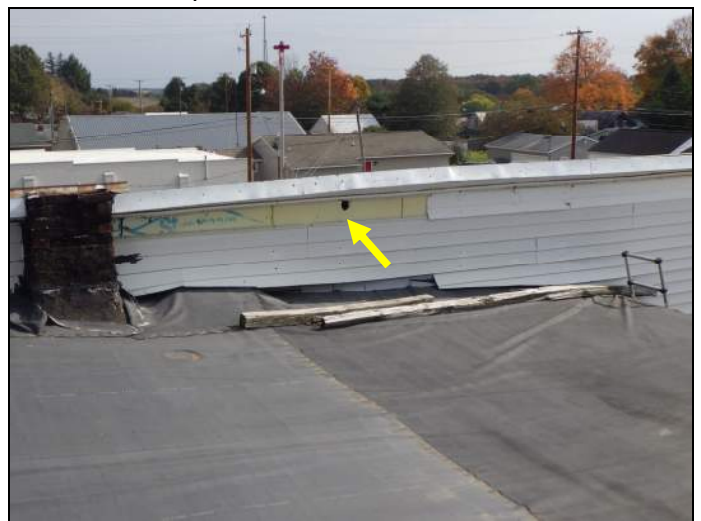
Missing vinyl siding
