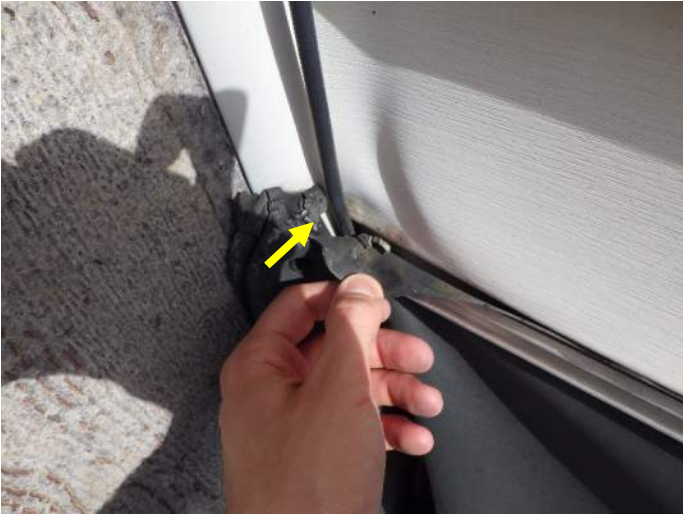
Void at corner in vinyl siding
