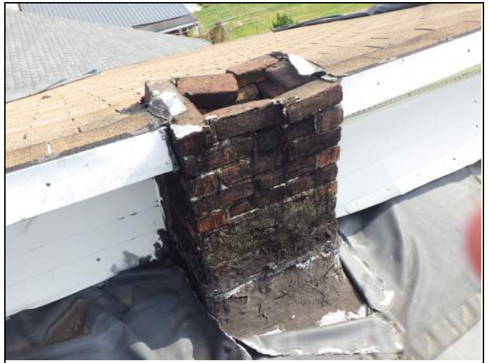
No termination bars or counter flashing at chimney
