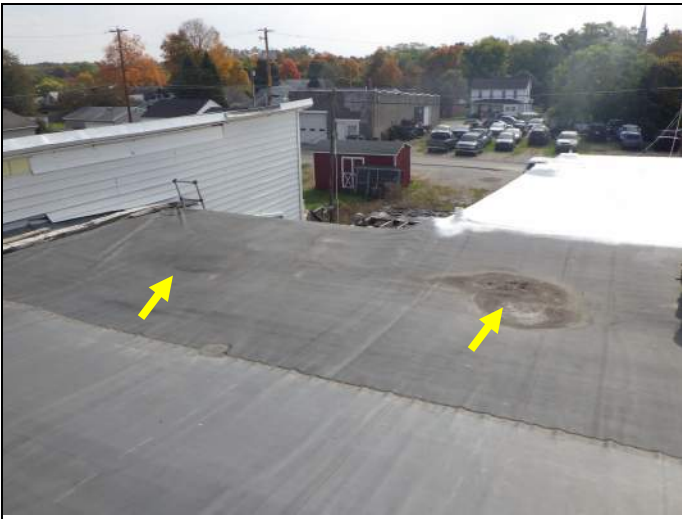
Low spots along south roof edge
