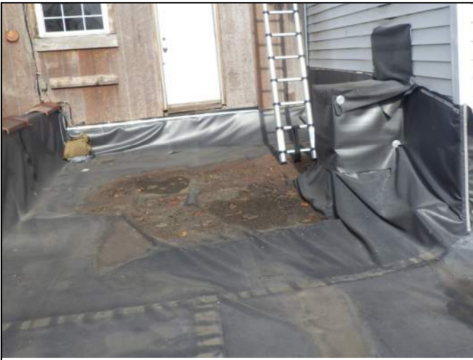
Dirt and debris on roof
