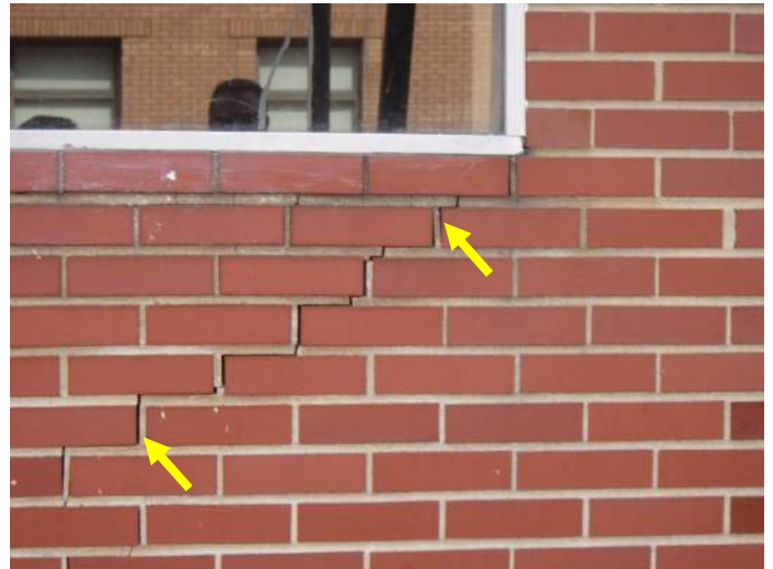
Incompatible mortar around window
