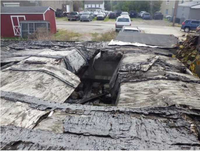
Deteriorated structure at rear
