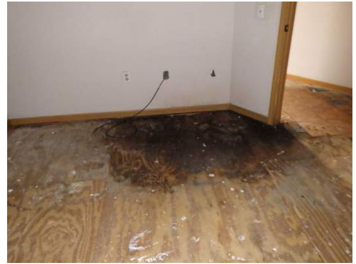
Area below water leak on second story
