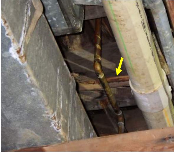
Fracture in second story floor joist
