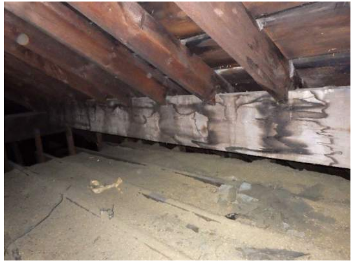
Water stains along beam in attic
