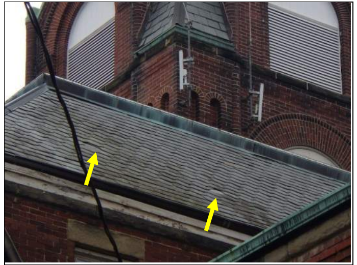
Fractured or missing slates
