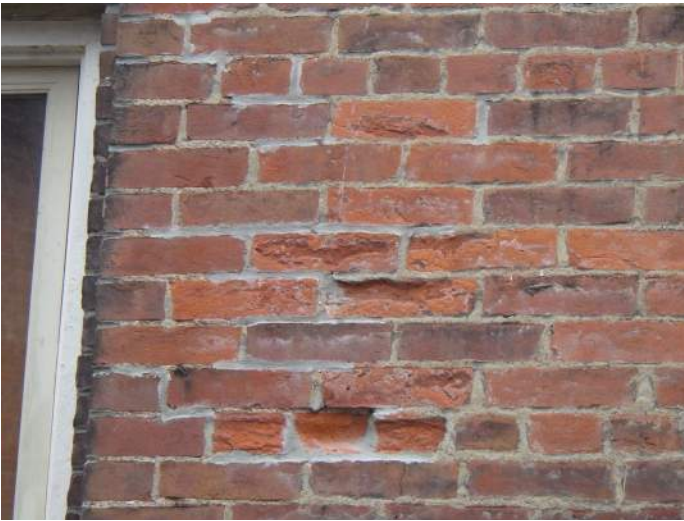
Spalled bricks at cementitious mortar
