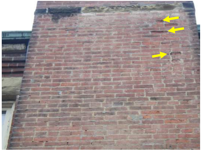
Spalled bricks at cementitious mortar
