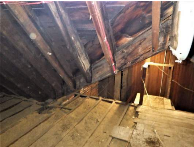
Water stains along valley rafter
