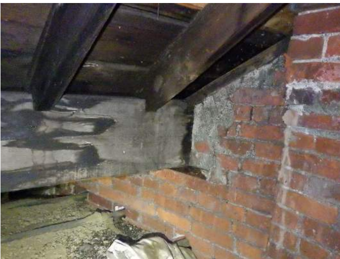
Water stains at beam support
