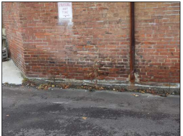
Stained and deteriorated bricks along alley
