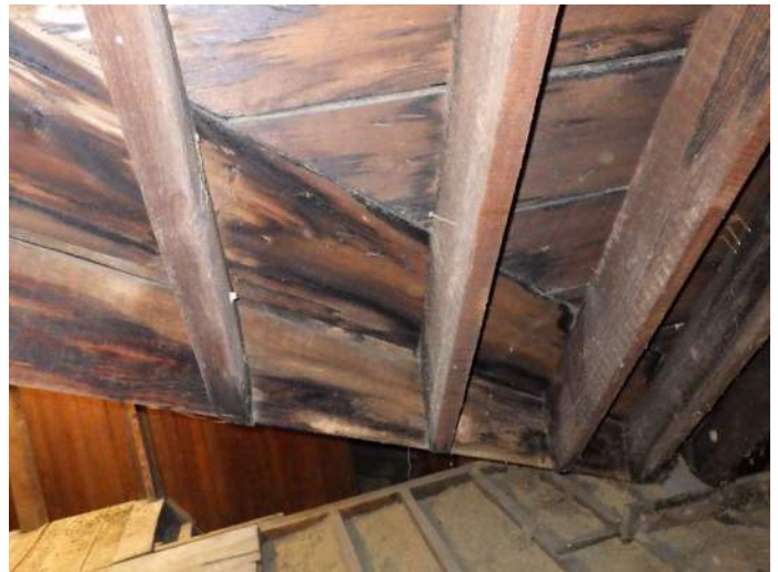
Water stains along valley rafter
