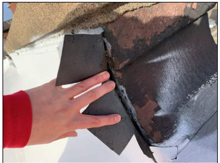
Loose roofing at parapet end
