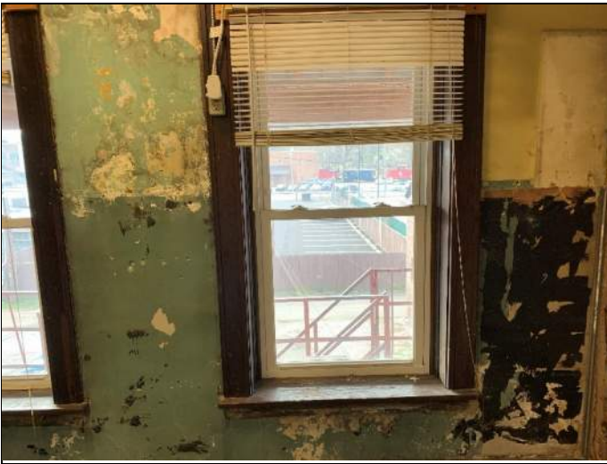
Wall condition at some residential apartments
