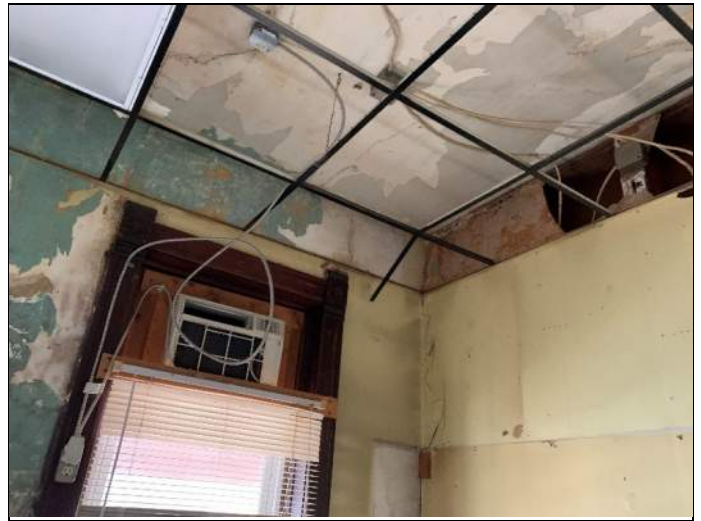
Wall condition at some residential apartments
