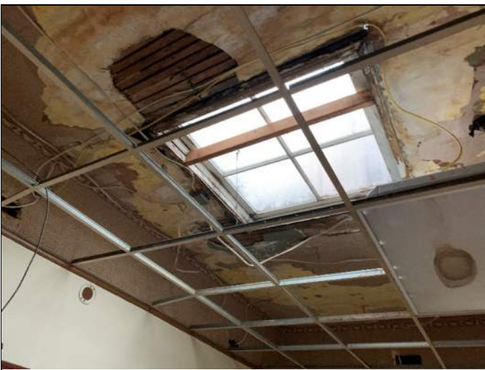
Ceiling condition at some residential apartments
