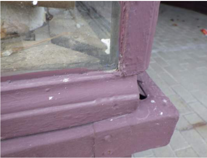
Typical window condition
