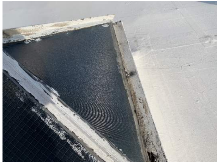
Condition of skylight
