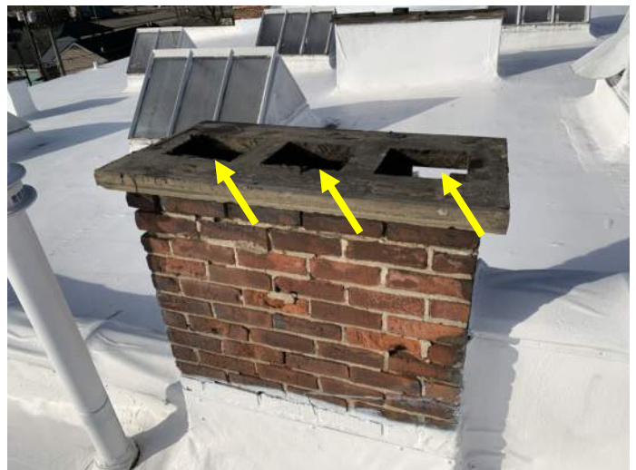
Absence of chimney flue caps
