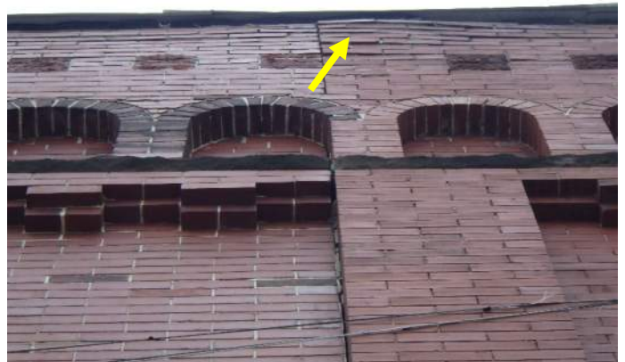
Brick wall bowing out above storefront
