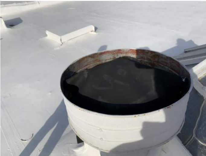
Vent missing hood covered with EPDM membrane
