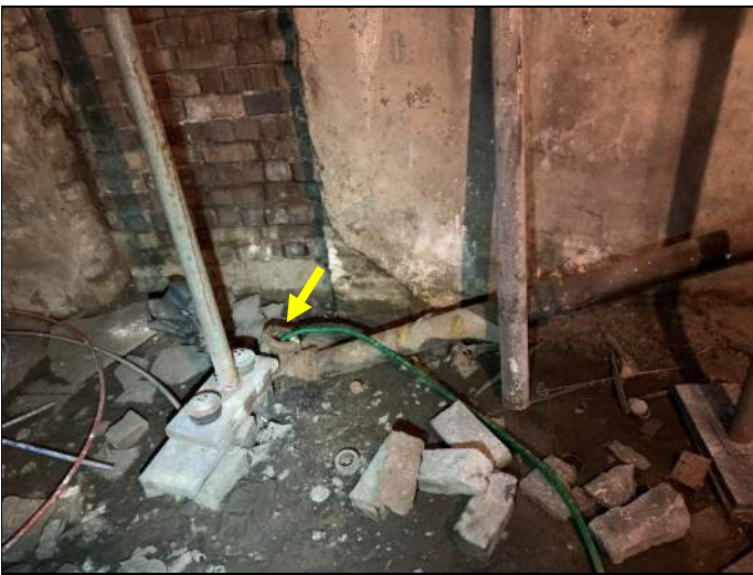
Waste water pipe with open fitting
