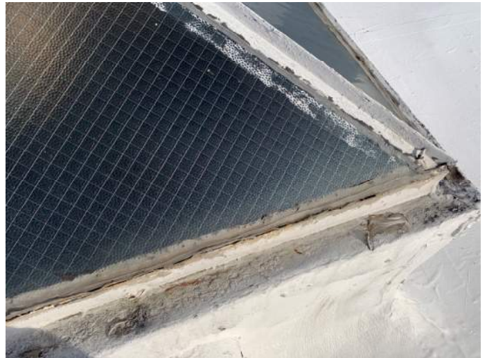
Deteriorated sealant along skylight joint
