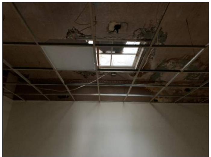
Ceiling condition at some residential apartments
