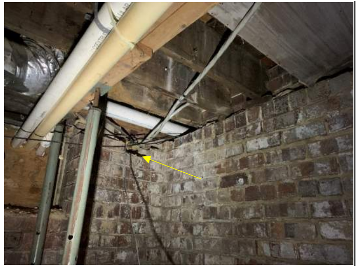
Deterioration of brick masonry wall
