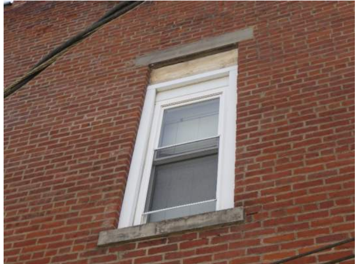
Typical vinyl framed window
