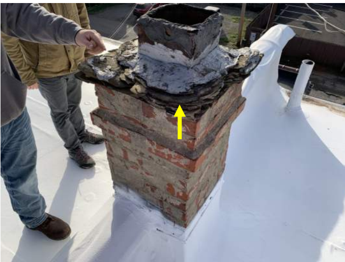
Deteriorated chimney crown
