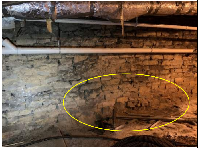
Deterioration of stone masonry wall
