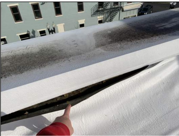
Loose and improperly overlapped roofing
