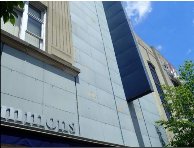
Paint flaking from metal panels
