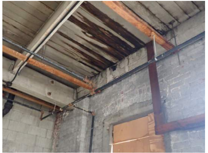
Typical water stains
