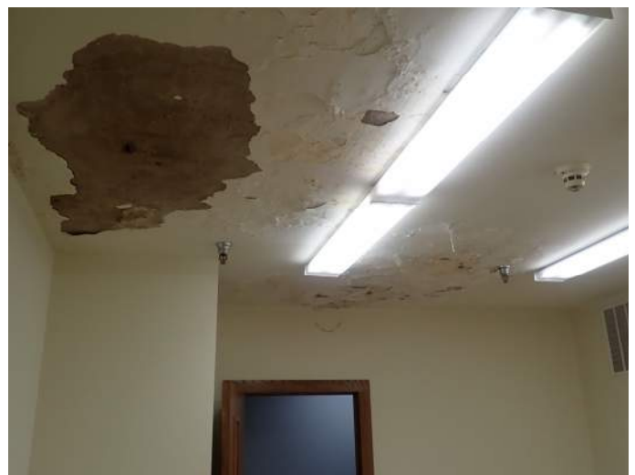
Stained second-story ceiling
