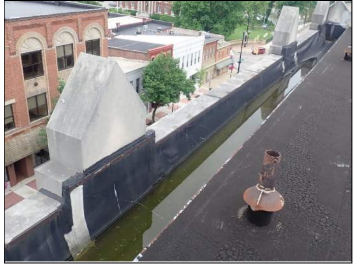
Clogged EPDM-lined gutter
