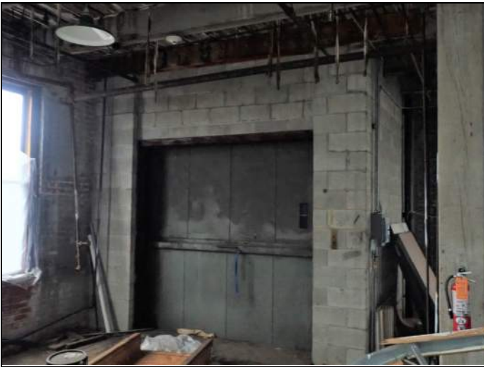
Service elevator at an upper story
