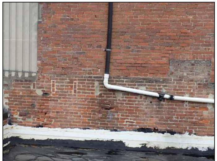
Damaged brick masonry
