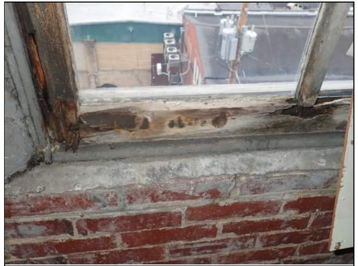
Typical window condition
