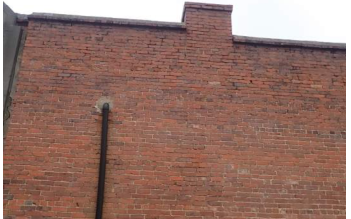
Deteriorated mortar between bricks
