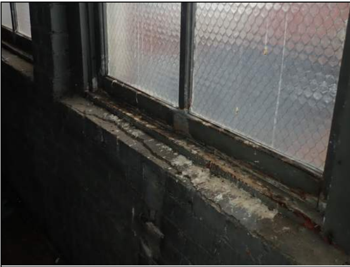
Typical window condition
