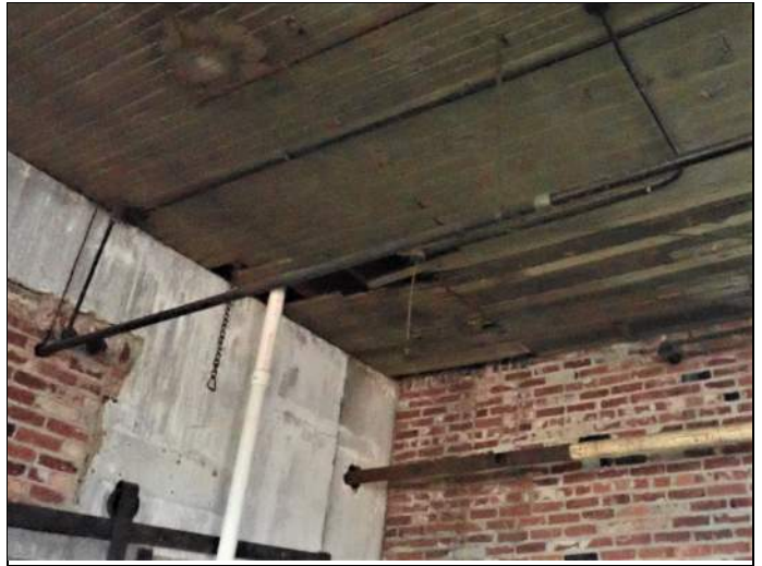
Water-stained ceiling panels
