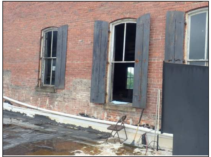
Typical window condition
