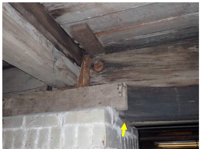
Crushed wood at support
