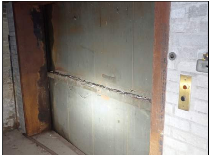
Service elevator in the basement
