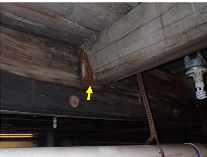
Corroded metal beam hanger
