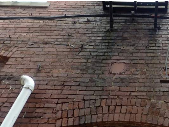
Deteriorated mortar between bricks
