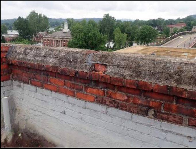
Deteriorated cement parge coating along top of parapet
