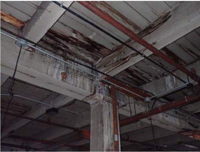
Typical water stains
