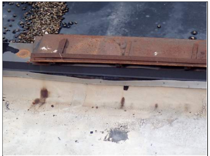
Loose metal flashing
