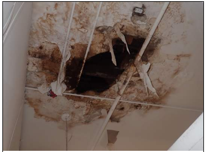
Stained ceiling and deteriorated roof framing
