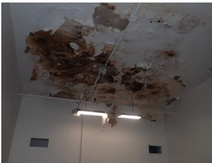
Stained third-story ceiling
